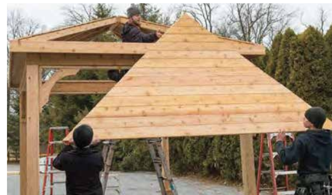
A) We notch the tops of your 6x6 posts 1 1/2" on both sides to fit your 2x8 beams, and B) we notch your 2x8 beams 1/2" deep to fit your 2x6 rafters
